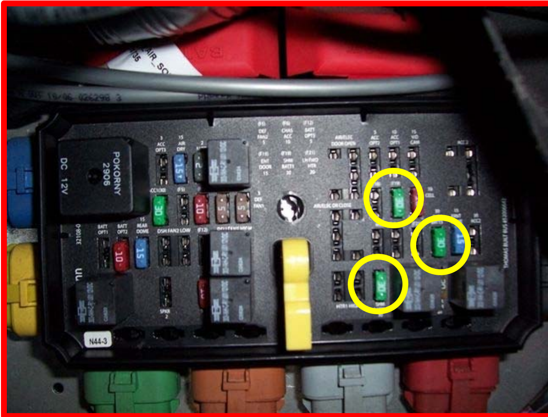
Photo 7: Photo shows the fuse block in driver's switch cabinet. Three 30amp fuses power the switch hub module (SHM). They are clearly labeled SHM.
