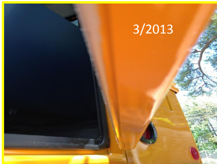
Bottom edge of exterior door after salt spray tests.
